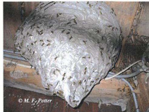
Fig. 7: Yellowjackets are one of the most dangerous insect pests in the U.S. Although nests are often constructed belowground, this one was located in an attic.
